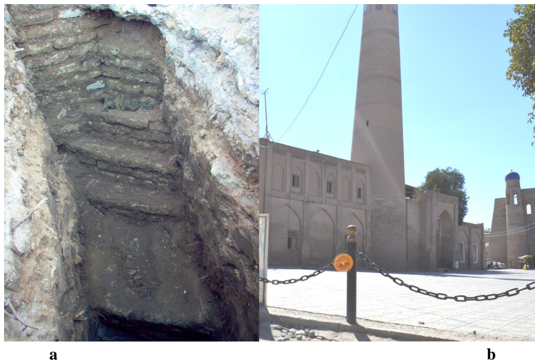
Figure 5. Basement of the minaret (a), Addressed to the department (Iron bars were placed) the deformation was stopped.
